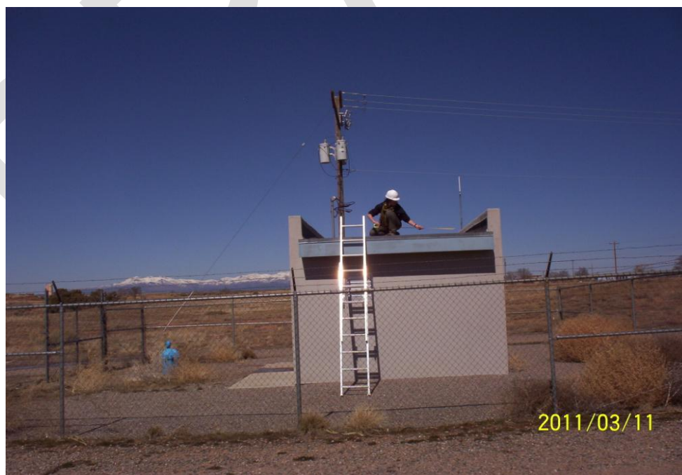
Installation of the meteorological station, North Pump House White Mesa, Utah.
