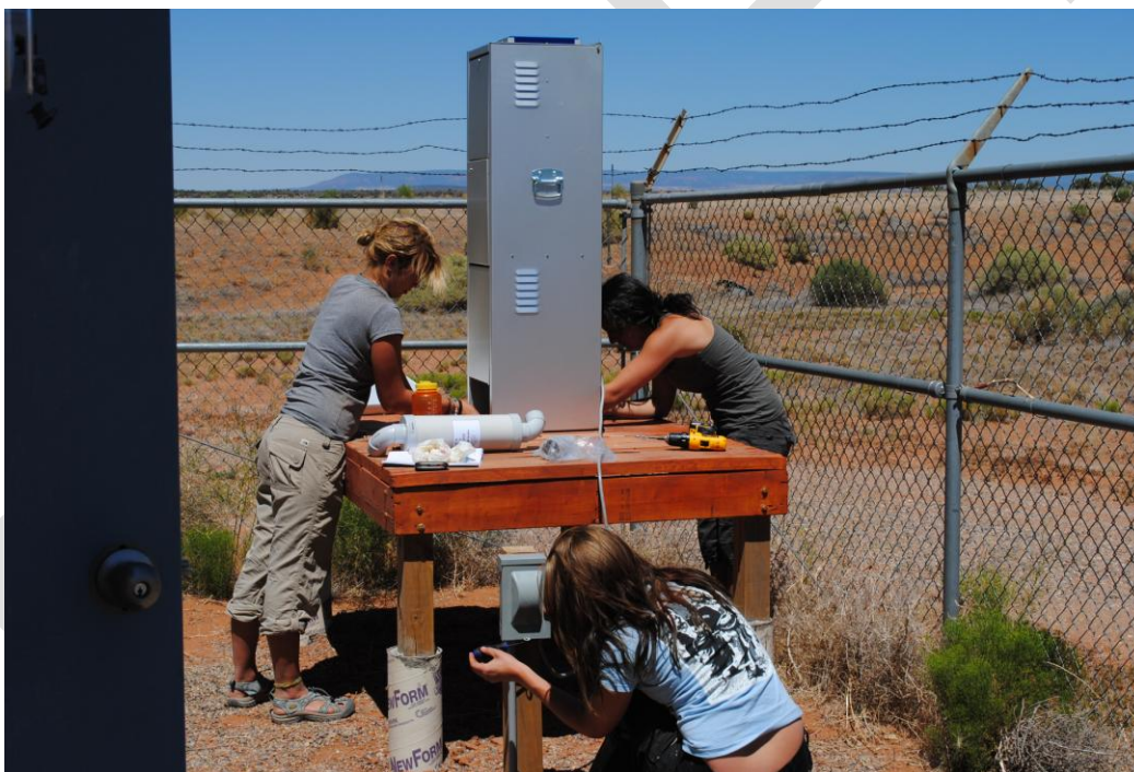
Installation of MV3000 in White Mesa, Utah.
