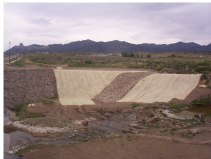
Navajo Wash erosion project
